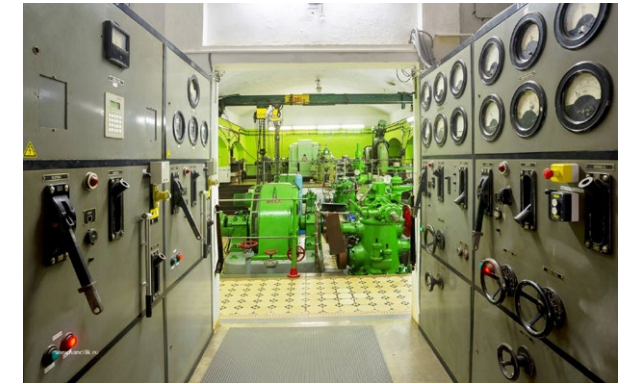
The distribution control panel for the generators
